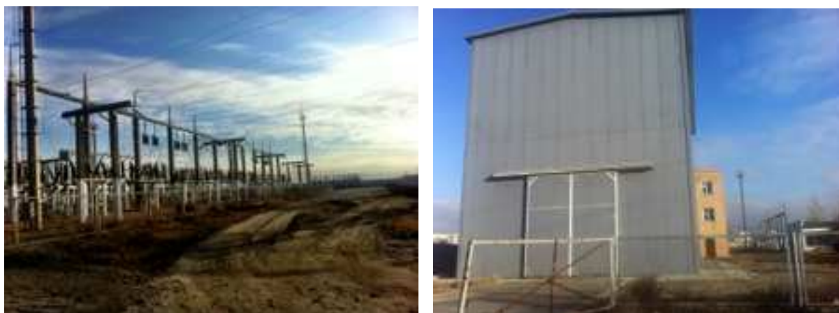
Location of the new PCB treatment facility at Tuul substation in Ulaanbaatar (9 October 2012)
